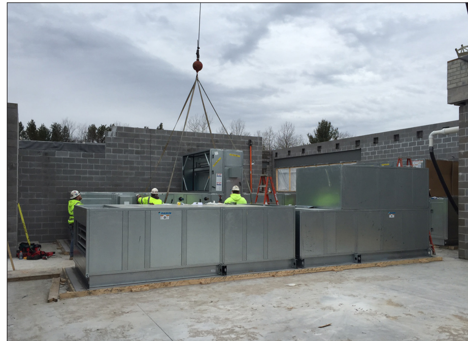
Second Floor AHU's
