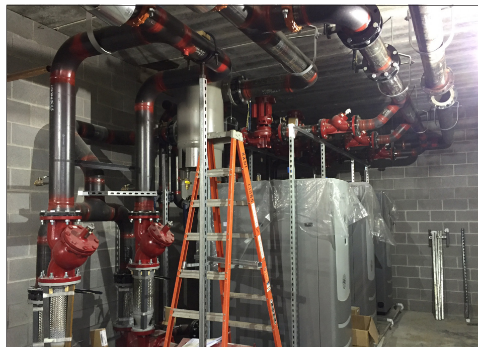
Boiler Room Equipment
